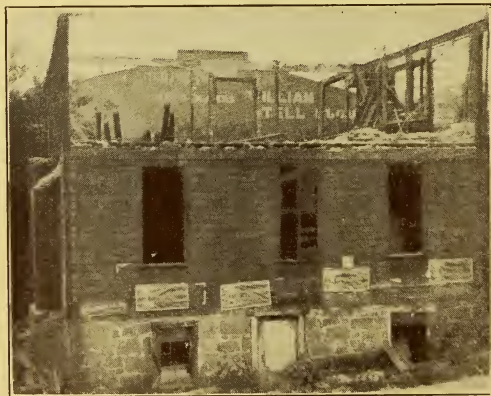
Unsafe building condemned by building inspector.
